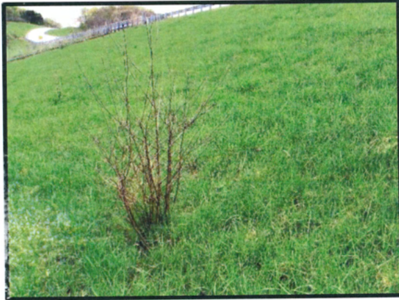
Fig. 31: Vegetation to be removed downstream west face
