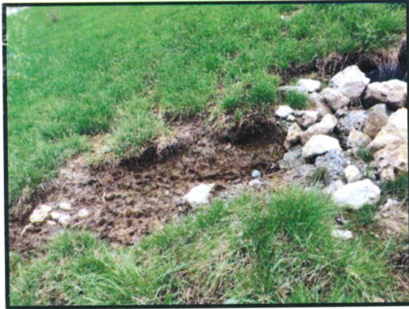
Fig. 25: Observed erosion at toe of aggregate roadway drain
