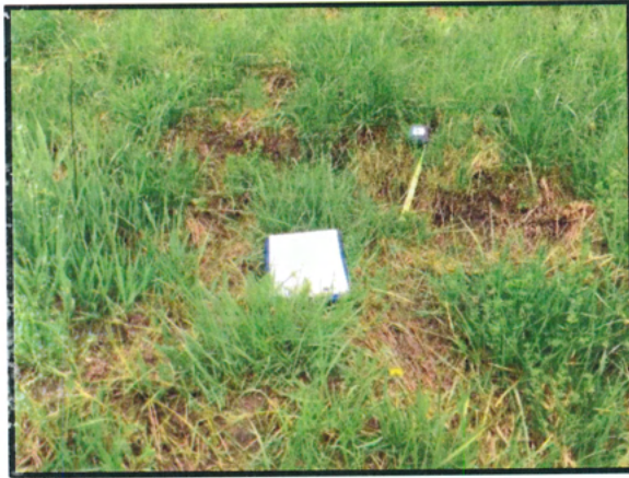
Fig. 39: Observed rutting east of spillway
