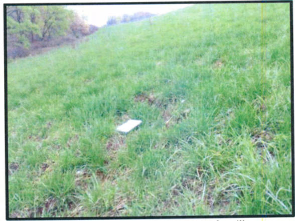
Fig. 40: Observed rutting east of spillway
