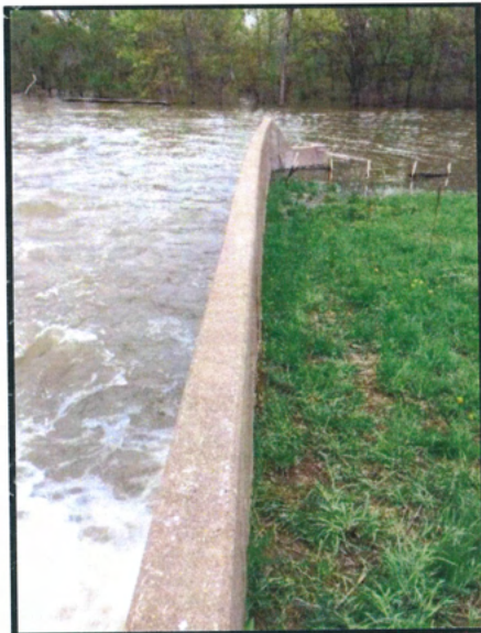
Fig. 37: East stilling basin wall bowing
