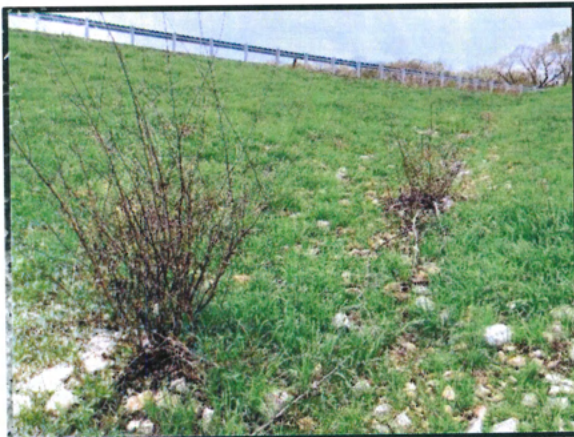
Fig. 23: Vegetation to be removed downstream west face
