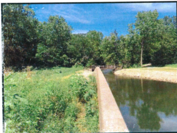
Fig. 49: West stilling basin wall bowing (Taken 08/01/2019)
