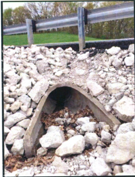
Fig. 17: Erosion at west roadway RCP armored with riprap
