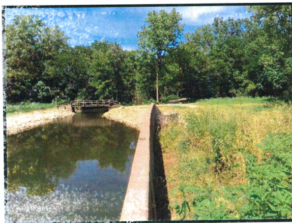
Fig. 43: East stilling basin wall bowing (Taken 08/01/2019)
