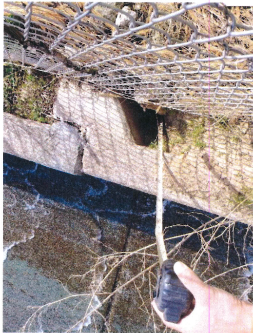
Figure 55: West joint G burrow to be filled
