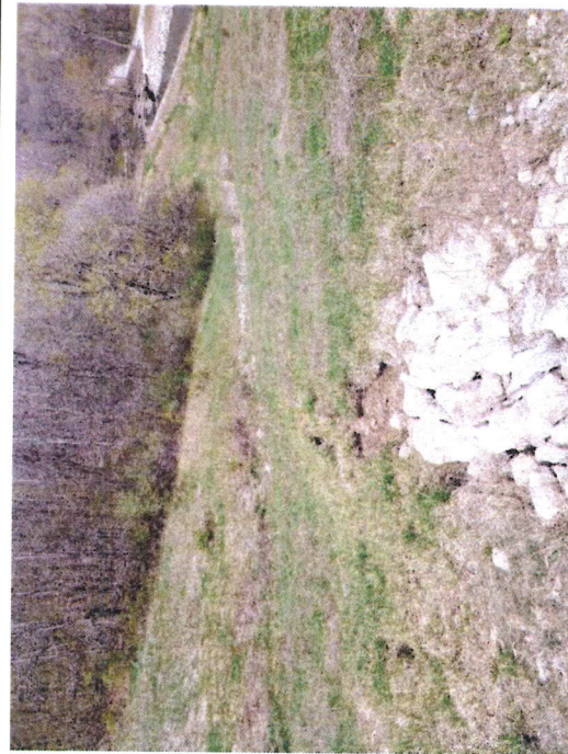
Figure 34: Adjacent erosion, west of spillway
