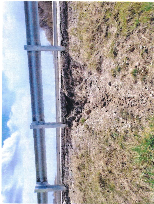
Figure 33: Shoulder erosion, west of spillway
