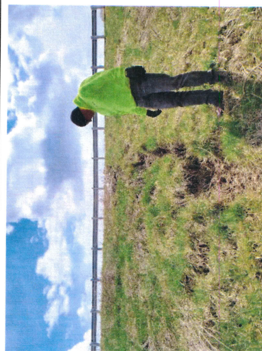
Figure 36: Continued erosion at downstream face, west of spillway
