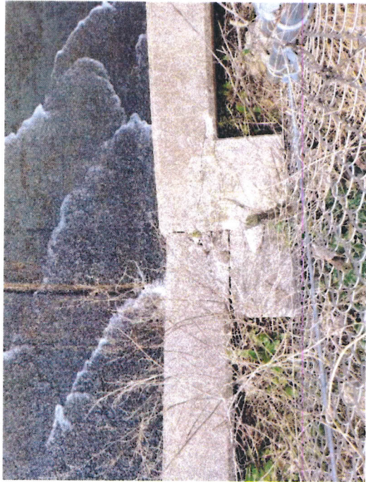
Figure 75: West spillway wall joint H
