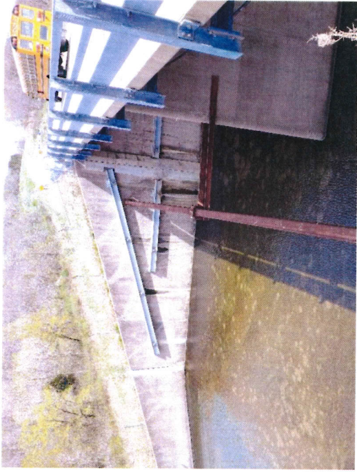
Figure 45: East spillway wall elevation w/ staining
