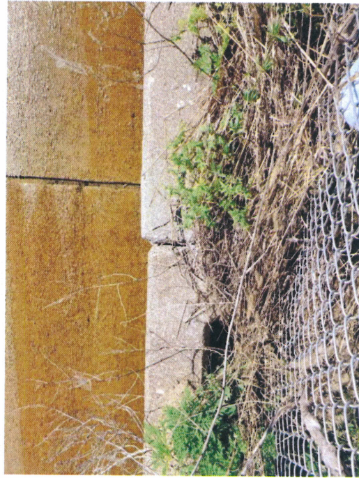
Figure 47: West spillway wall joint G
