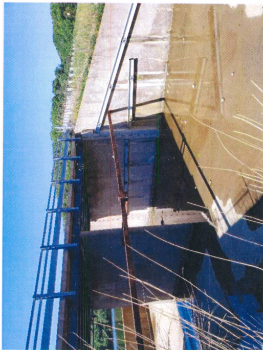
Figure 73: West spillway wall elevation w/ staining
