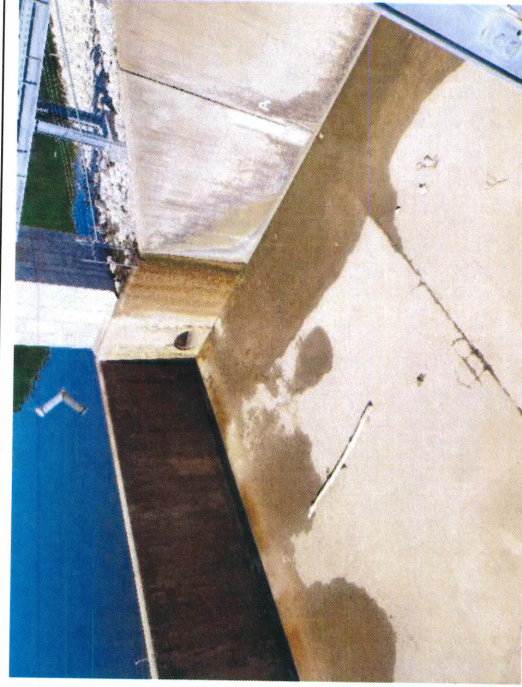
Figure 12: Dewatering structure, sluice gate, floor slab cracks (NC)
