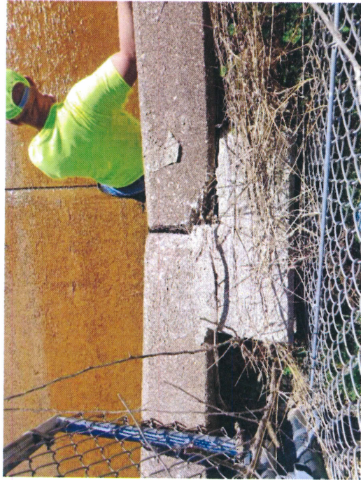
Figure 49: West spillway wall joint H
