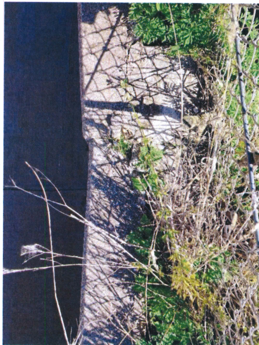
Figure 61: West spillway wall joint H
