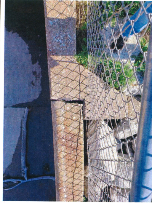
Figure 14: East spillway wall joint A cracking
