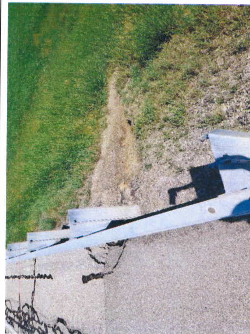
Figure 32: Shoulder erosion, west of spillway
