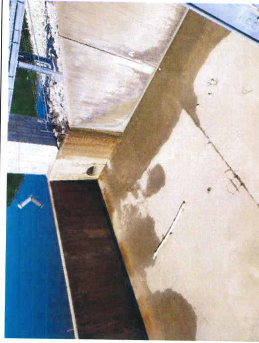
Figure 12: Dewatering structure, sluice gate, floor slab cracks (NC)
