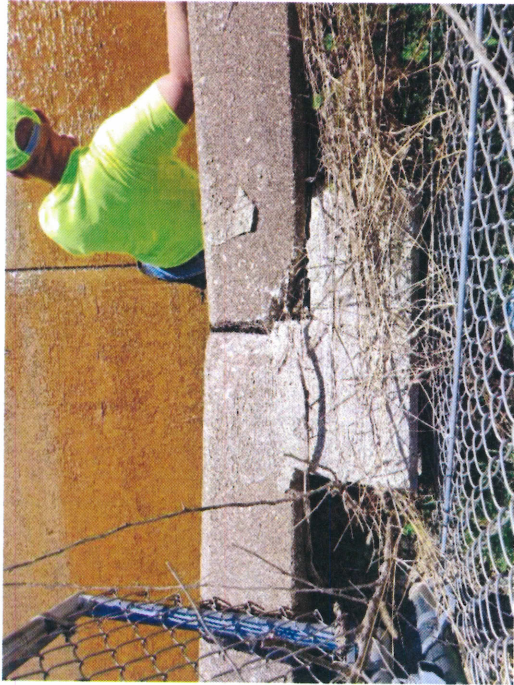
Figure 49: West spillway wall joint H
