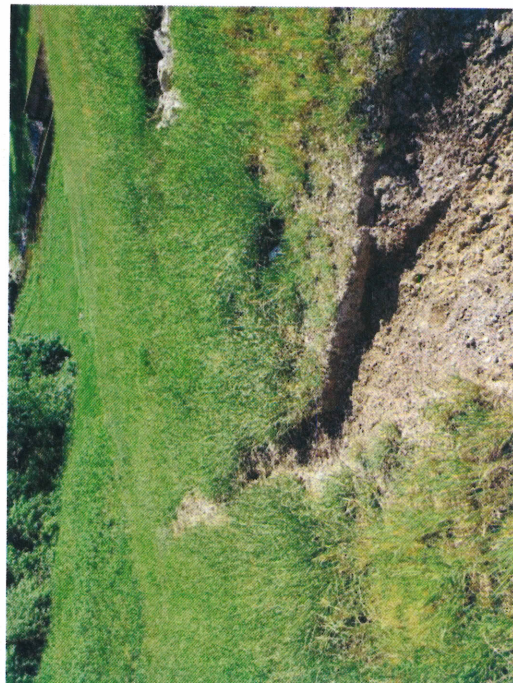
Figure 31: Shoulder erosion, west of spillway
