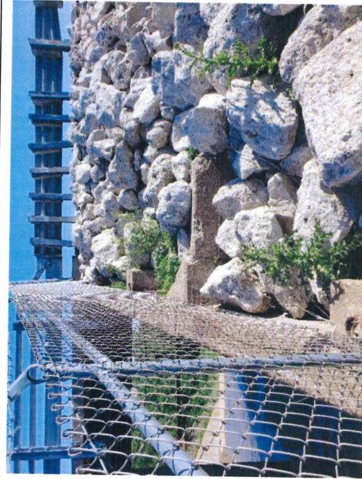
Figure 11: Southeast spillway wall wing crack
