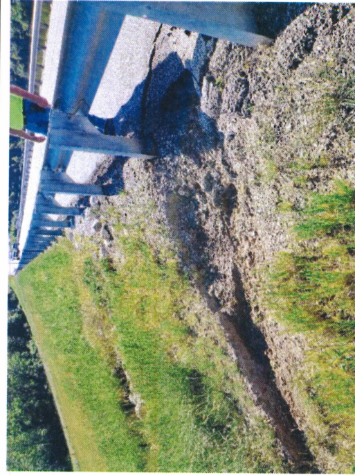
Figure 30: Shoulder erosion, west of spillway
