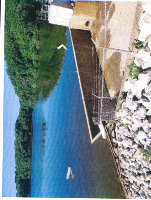
Figure 8: Spillway and warning buoys
