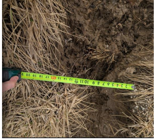
Figure 31: Erosion Rill, West of Spillway
