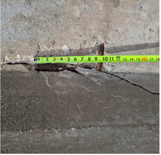
Figure 60: East Spillway Wall Exposed Rebar, No Change
