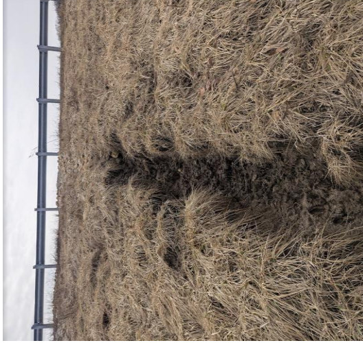
Figure 30: Shoulder Erosion Rill, West of Spillway
