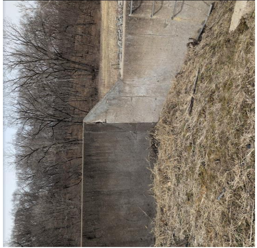
Figure 59: East Spillway Wall Crack, No Change
