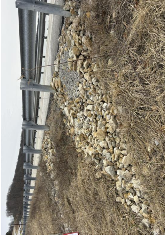
Figure 27: Shoulder Erosion Fill-in, West of Spillway
