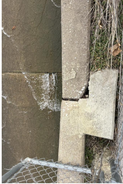
Figure 51: West Spillway Wall Joint H
