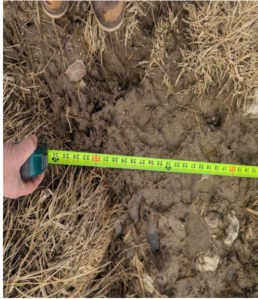
Figure 33: West Downstream Slope Erosion Rill
