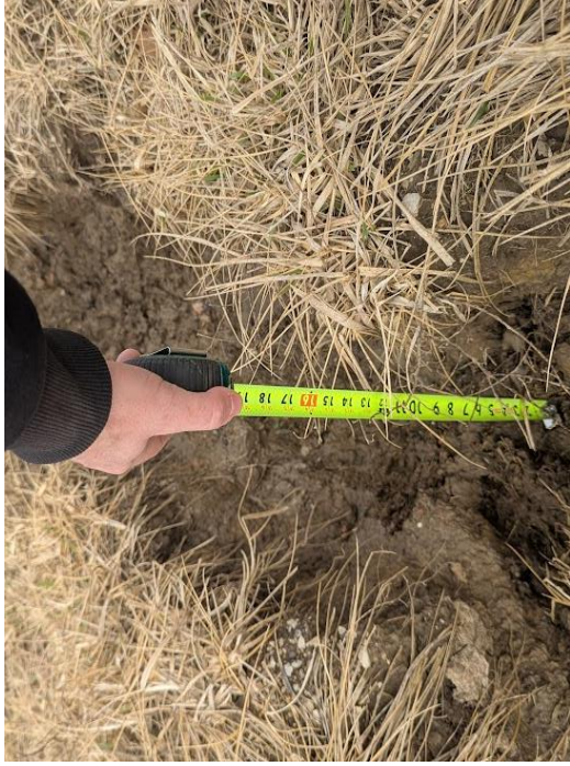
Figure 34: West Downstream Slope Erosion Rill
