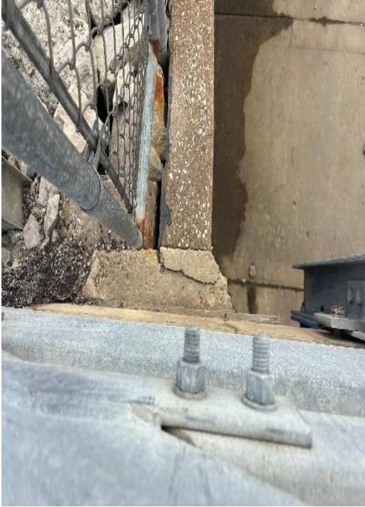
Figure 9: Spall at Southeast Bridge Abutment/Spillway Wall Corner
