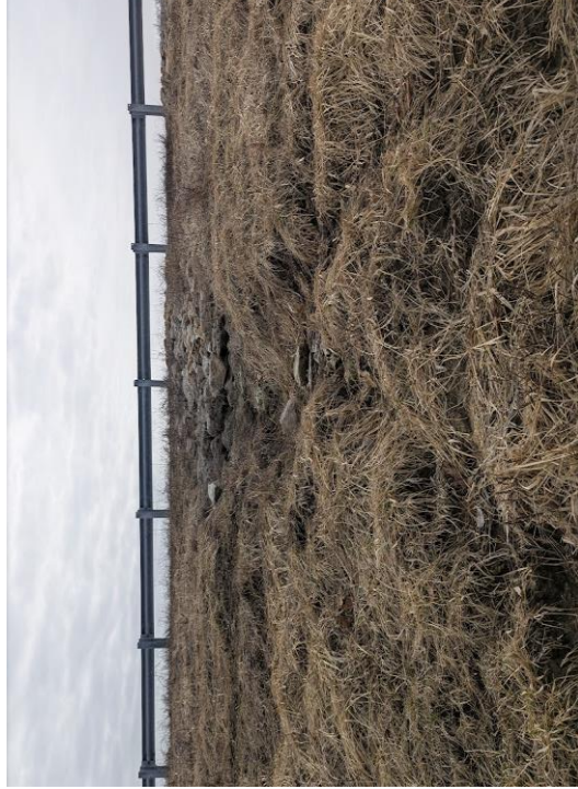
Figure 29: Shoulder Erosion, West of Spillway
