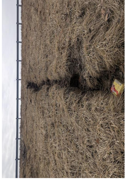
Figure 32: Continued erosion at downstream face, west of spillway
