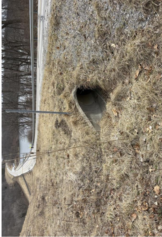
Figure 25: West Roadway RCP Inlet End Section
