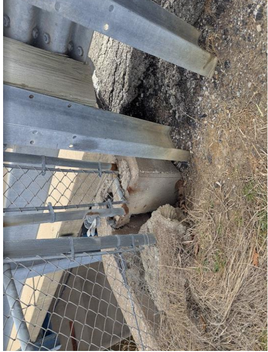
Figure 37: Loss of Material Behind West Abutment along North Shoulder
