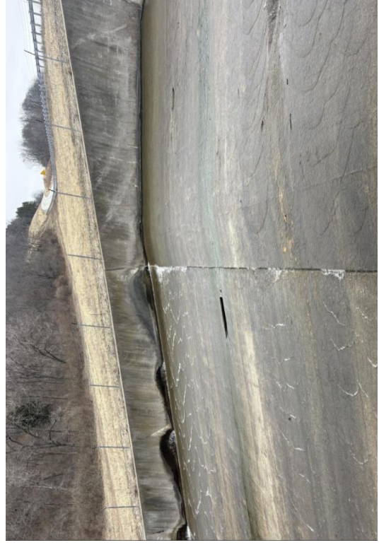
Figure 40: Active Drainage through Floor Joints
