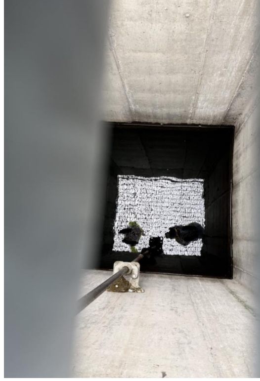
Figure 20: Dewatering Structure Interior / Operating Stem
