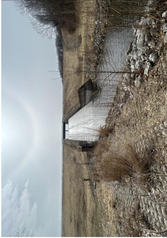
Figure 57: Outlet Works Woody Vegetation
