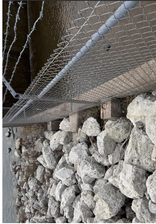
Figure 13: East Spillway Wall Joint A Crack
