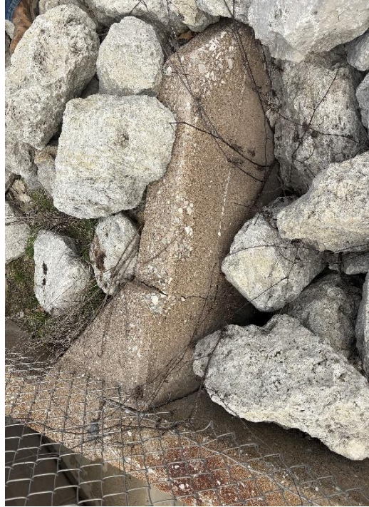
Figure 11: Southeast Spillway Wing Wall Crack
