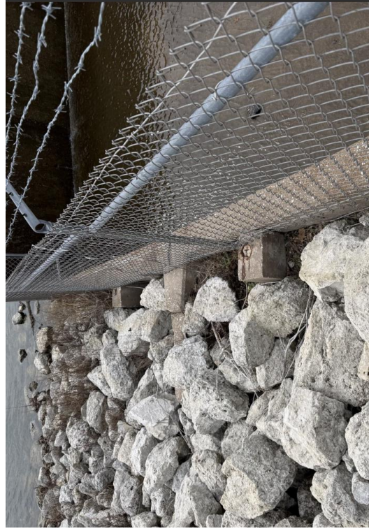
Figure 13: East Spillway Wall Joint A Crack
