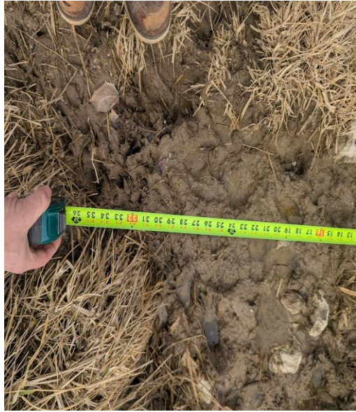
Figure 33: West Downstream Slope Erosion Rill
