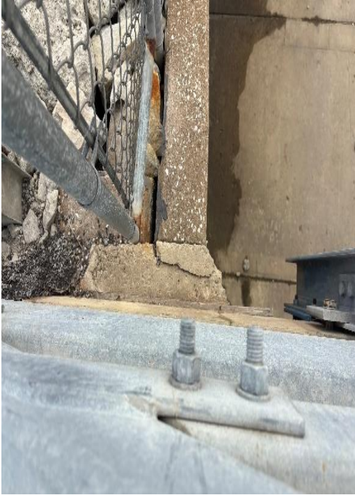
Figure 9: Spall at Southeast Bridge Abutment/Spillway Wall Corner
