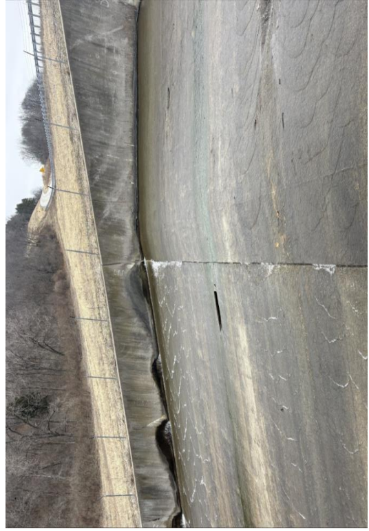
Figure 40: Active Drainage through Floor Joints
