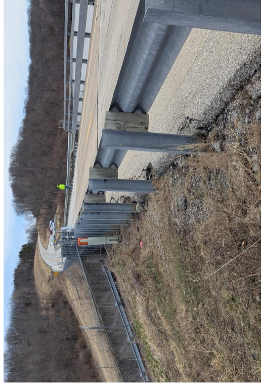
Figure 79: Longitudinal and Transverse Cracking on North Shoulder
