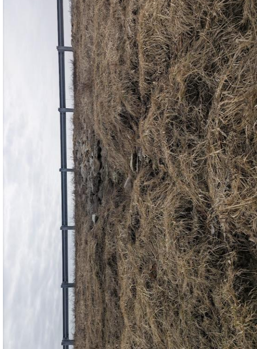
Figure 29: Shoulder Erosion, West of Spillway
