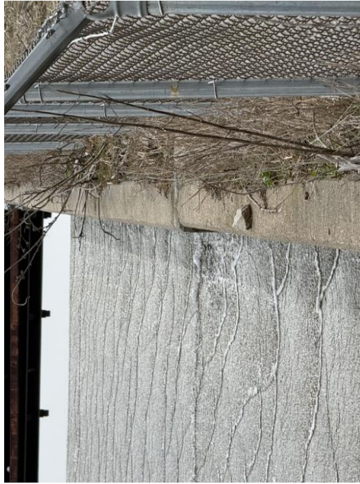
Figure 49: Slight Outward Movement of Wall from Joint F to G
