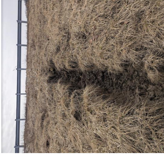
Figure 30: Shoulder Erosion Rill, West of Spillway
